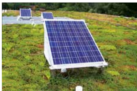
The test involved two modules installed on a “naked” membrane panels being compared with one module installed on a green roof. In each case, attention was focused on the temperature at the underside of the panels.
