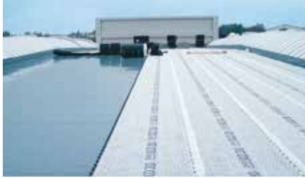
1. The roof membrane is covered with the protection, drainage and water retention element Fixodrain® XD 20.
