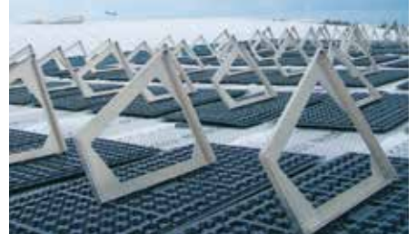
3. The Solar Base Frames SGR are placed and adjusted on the ZinCo Solar Bases.
